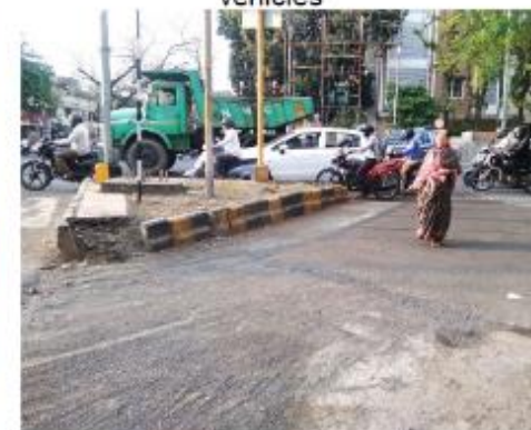
Underutilized refuge island with no access for pedestrian
